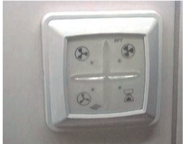
Figure 3. Ventilation controller without guidance on its standard setting nor feedback on which setting it is on.
